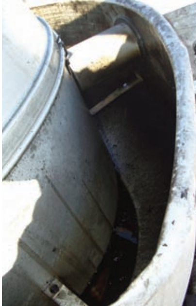
Typical extractor, 3 months since prior cleaning. Notice the accumulation of grease liquids in the bottom of the extractor.
