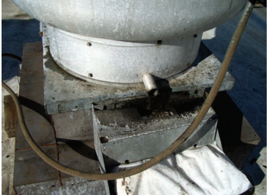
Another typical extractor with overflow discharge, 3 months since prior cleaning. Notice the overflow has spilled onto the roof area around the extractor.
