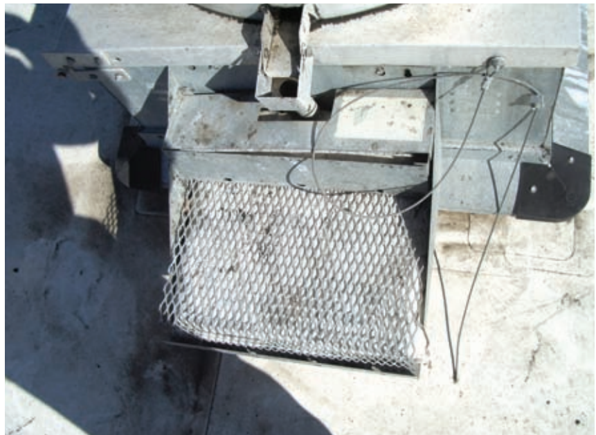
Applebee's Murrieta extractor with the new system, 6 months since prior cleaning. Notice there is no overflow 6 months after prior cleaning — the roof area around the extractor remains grease free.
