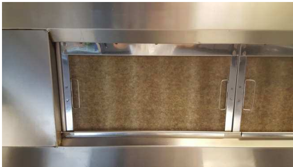
Filters starting to show grease accumulation. Notice the “ribs” of the baffle filter becoming visible.
